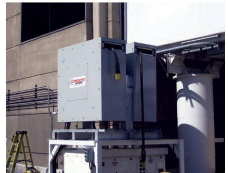
PLB400 mounted at the tarmac level and suspended above the converter.
