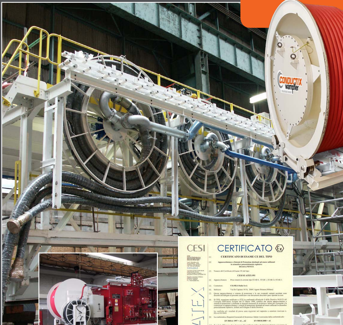
24kV reel with ATEX slirping
