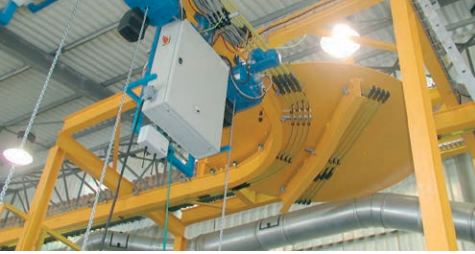
SinglePowerLine 0812 in a galvanizing plant with bridge elements on a turning gate and dual collector assemblies
