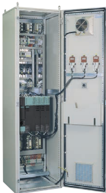
Control panel with variable frequency drives for three motorized trolleys – by Conductix-Wampfler
