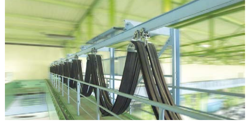
On the go! Program 0350 cable trolley system on a steel mill overhead bridge crane
