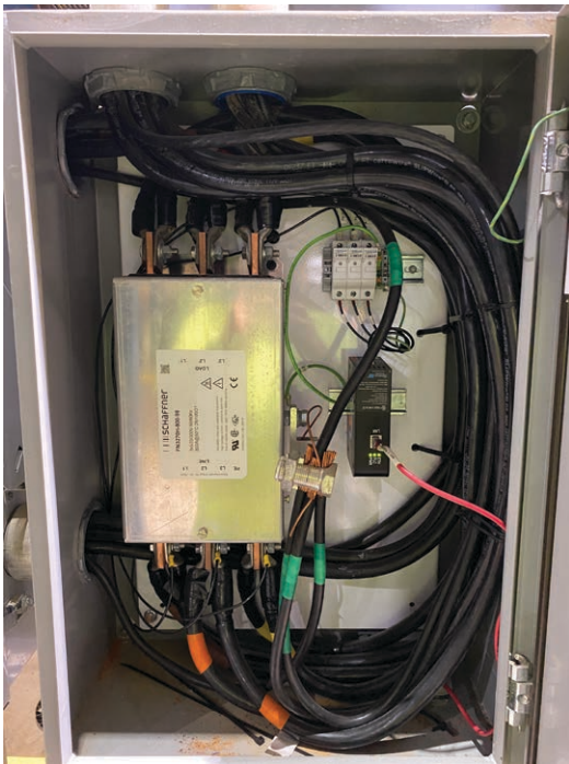
Figure: 6-6 - Improper Installation of System
